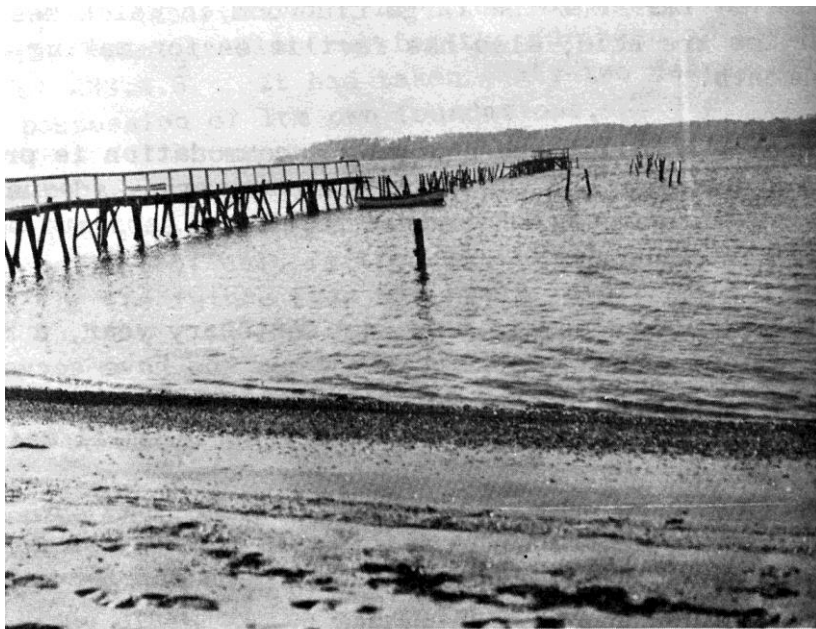
Gale damaged pier, 25 October 1937
